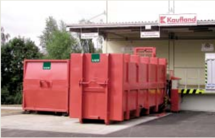
Stationary compactor and press container near the ramp - outside installation (Kaufland)
